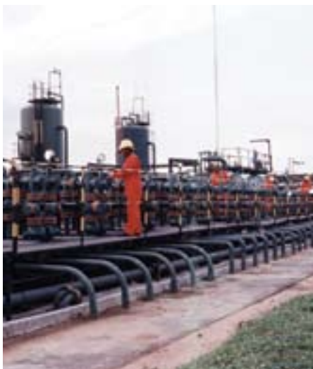
• SPDC: Obigbo North flowstation
